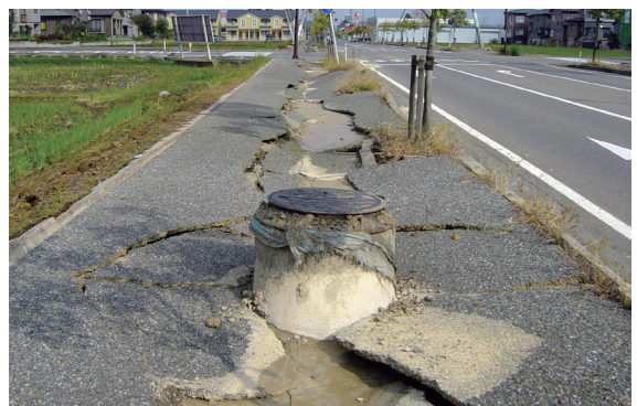
Roads damaged in the Chuetsu earthquake in Japan on October 23, 2004 © Tubbi
